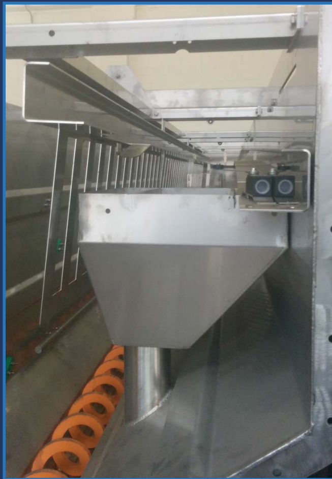
Floatings collection system
