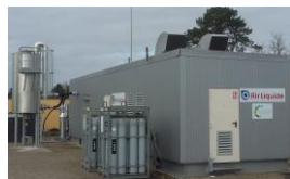
Biogas upgrading with membranes
