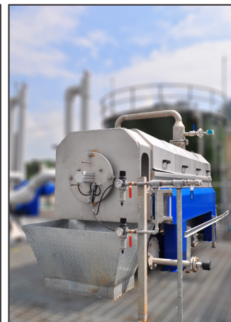
An SSD installation
